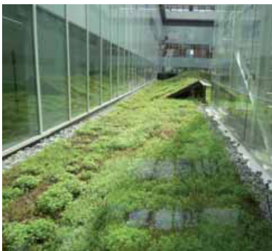
Green roof with C2C system Location: Mollet Hospital, Barcelona Project: Coreia Moran - Alex Puig Customer: Mollet Hospital
